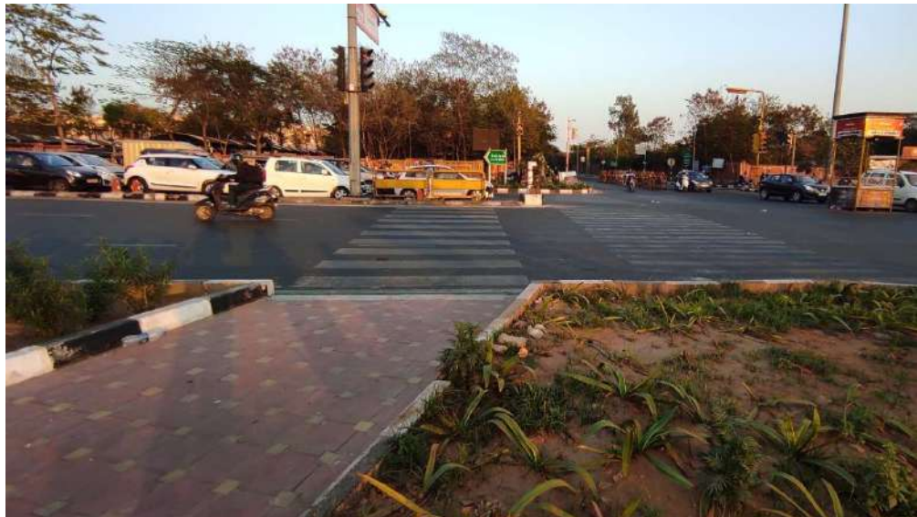
Figure 20: Faded and Improper demarcation of Zebra crossing
